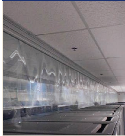
PHOTO 1 Separation of detection and suppression from aisle containment.
