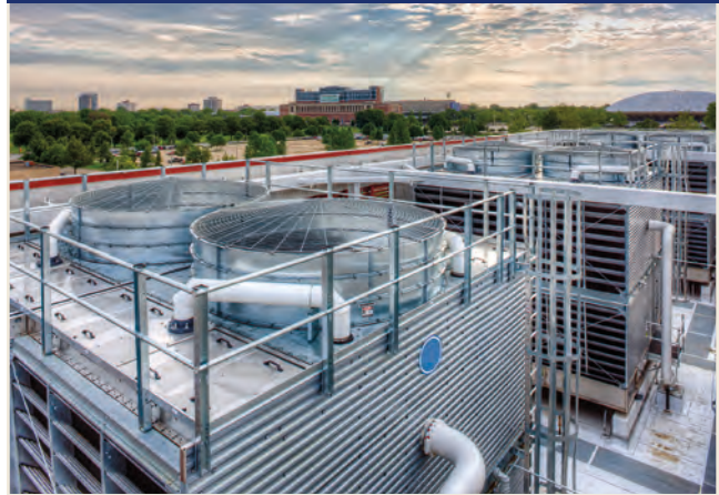
PHOTO 2 Open circuit cooling towers on a liquid-cooled data center. Courtesy of National Center for Supercomputing Applications (NSCA)
